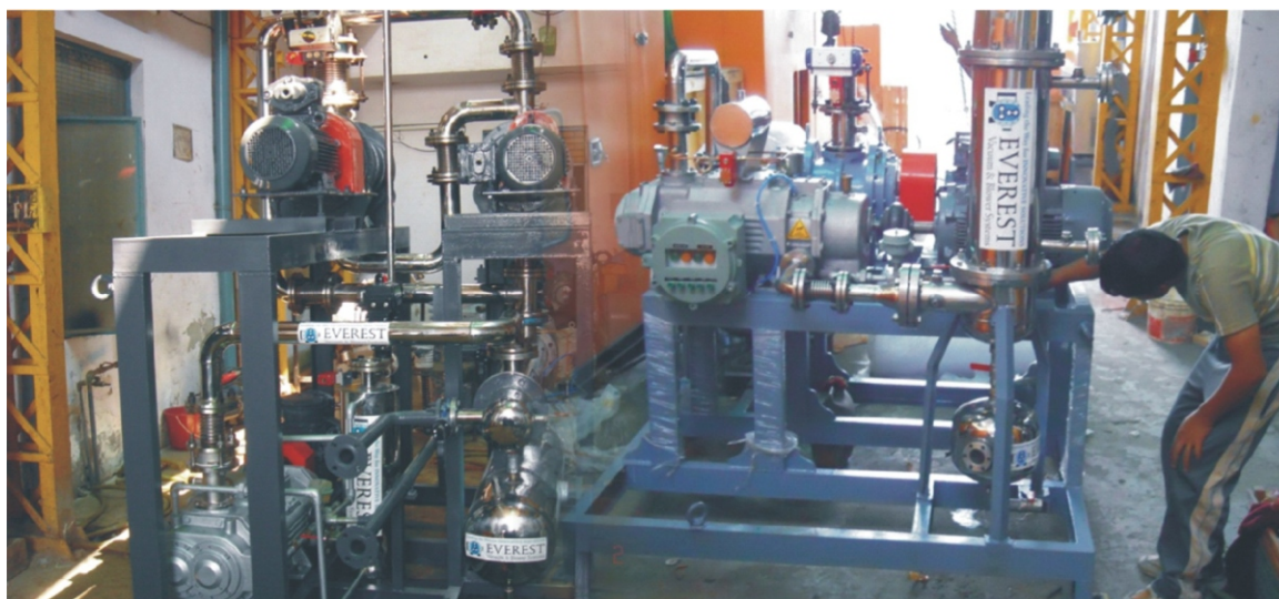
Fig: Vacuum system supplied to a pharmaceutical company in Visakhapatnam.
