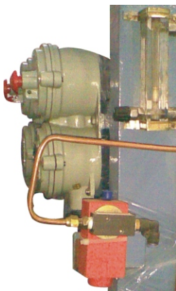
Fig: Solenoid Valve for Nitrogen Purging with Rotameter
