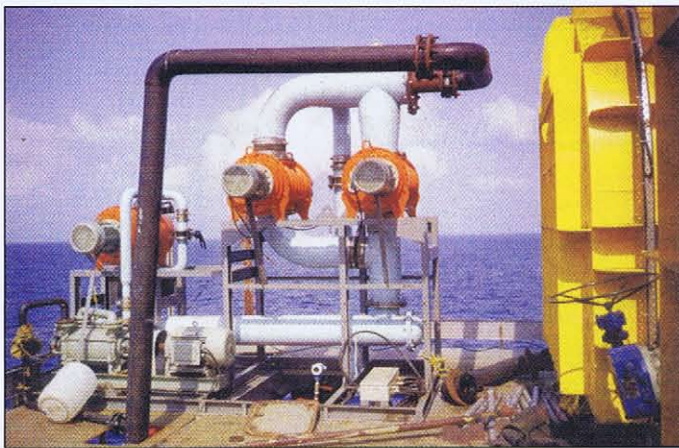
De-aerator and condenser vacuum systems supplied by Everest Transmission, New Delhi
