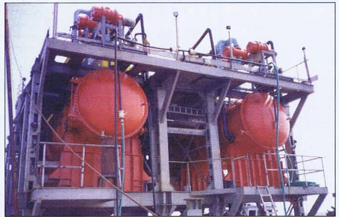
Condenser of the floating barge mounted LTTD
