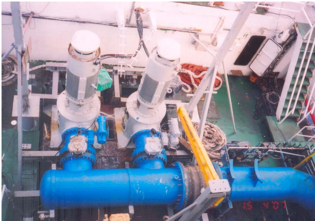
Fig 10: Warm Water Pumps of the Floating Barge Mounted Desalination System
