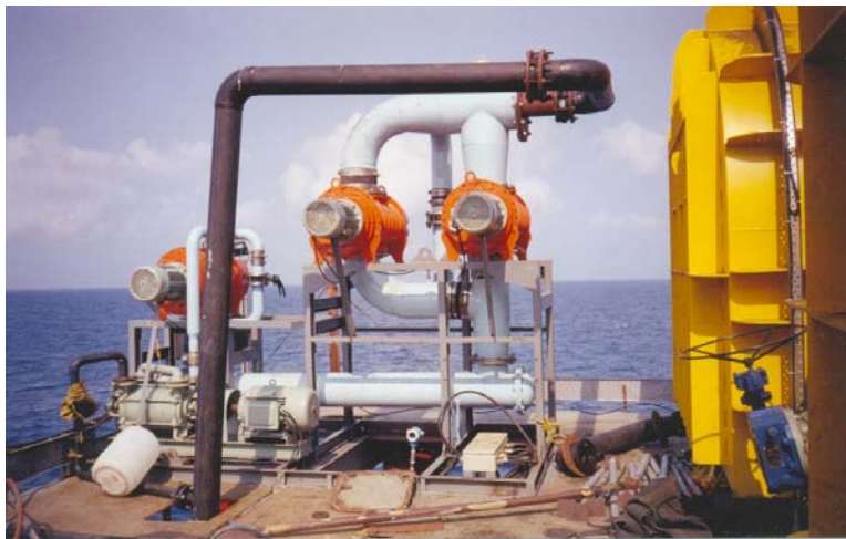
Fig 11, 12 & 13: De-aerator & Condenser Vacuum Systems supplied by Everest Transmission, New Delhi.
