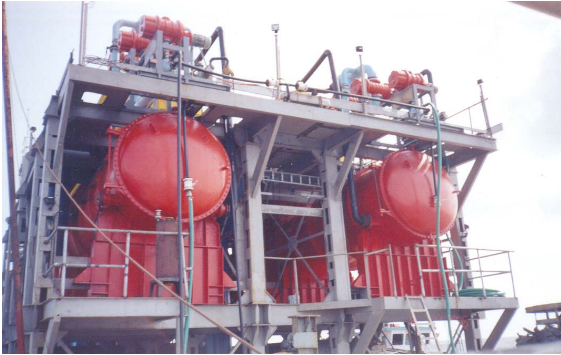
Fig 17: Condenser of the Floating Barge Mounted Low Temperature Thermal Desalination Plant
