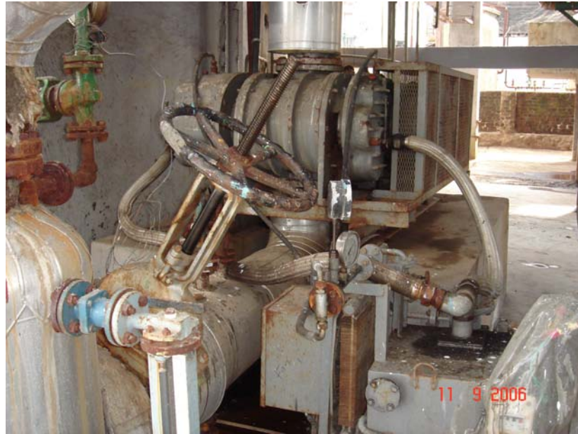
Fig 8: Typical Everest Mechanical Vapor Compressor Installation
