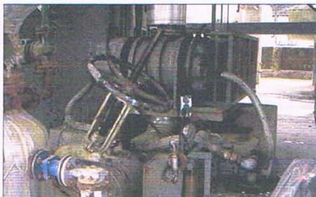
Fig 8: Typical Everest Mechanical Vapor Compressor Installation
